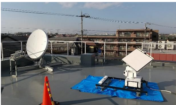
Figure 2: Gateway station and VSAT station.
