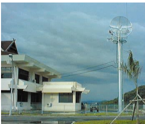
Bili Bili Dam Telemetry System (Indonesia)
