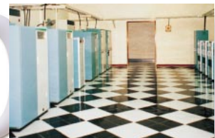
Vietnam Coastal Communication System Hai phong- Transmitting
