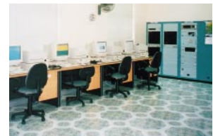
Vietnam Coastal Communication System Hai phong- Operation Center
